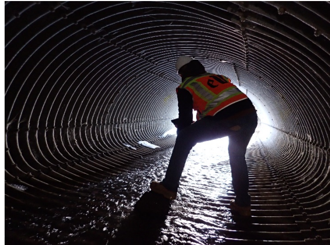
Figure 5-1: CMP Culvert. Source: Engineering Operations.
